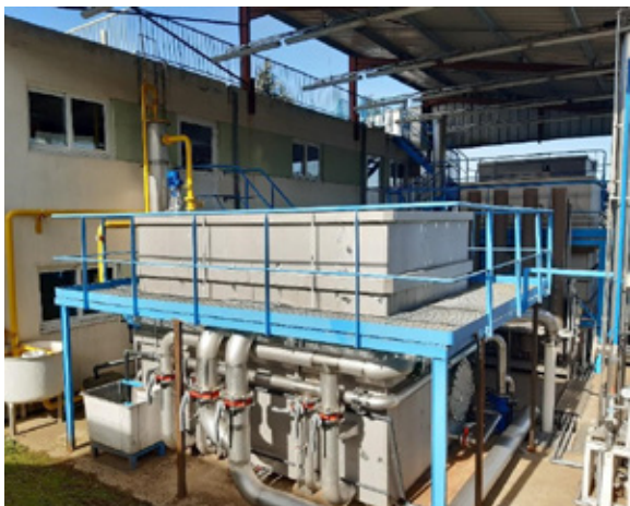
New compact drinking water treatment plant - OiEau Training Centre - La Souterraine site. ©OiEau
