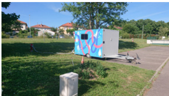
Pressurising the leak detection network with the INRAE mobile unit, designed by OiEau in 2020. ©OiEau
